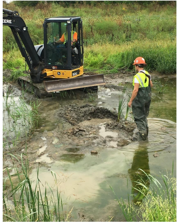
Figure 15 Bioretention Not Draining
