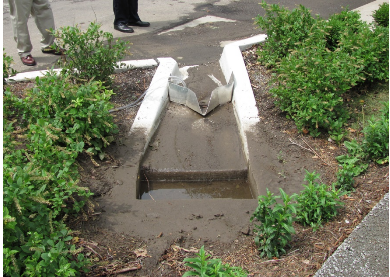
Figure 3 Inlet Flow Monitoring
