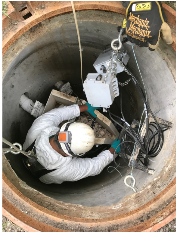
Figure 1 Space Constrained Meter Installation
