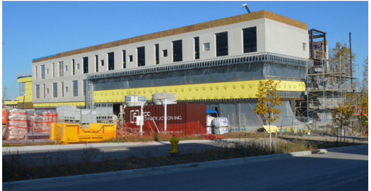
The school is built into a hillside between Grandville Avenue SW and the U.S. 131 freeway
