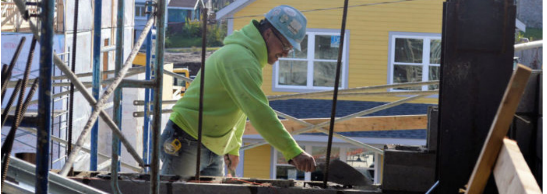
Tim Horton of JK Masonry lays concrete block in the south wall of the new
