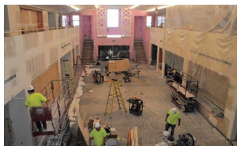
Workers are transforming the former museum at 54 Jefferson Ave SE into a new high school of Grand Rapids Public Museum
