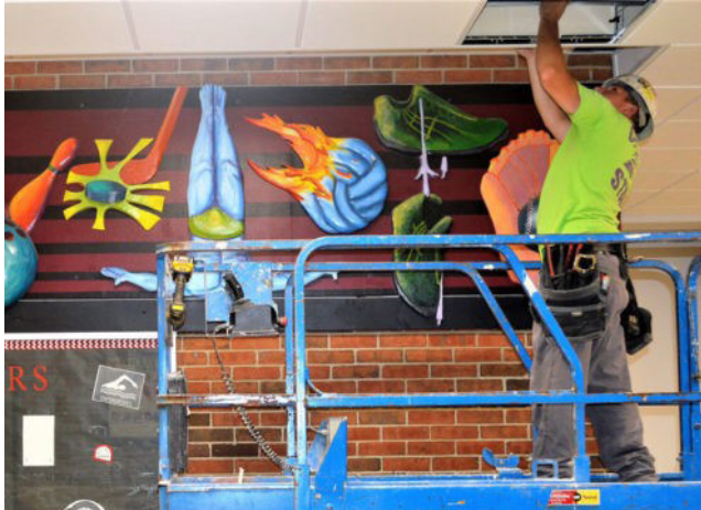
Pat Doane of the Schepers Brothers Co. installs new ceiling tile in the lobby outside the Union High gymnasium.
