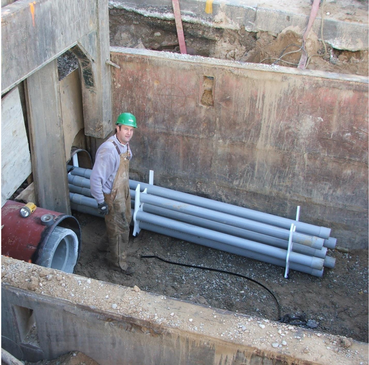
P5 Duct alongside Storm Sewer under US131
